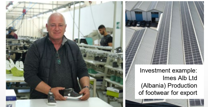
Financed installation of 0.5MW rooftop solar panels to cover all its own electricity needs
